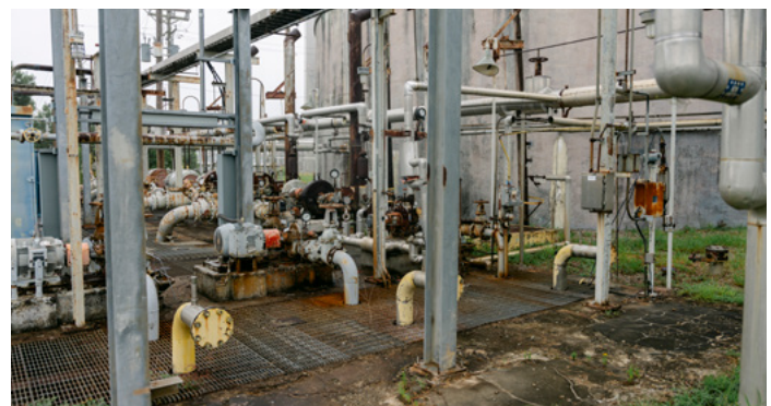
BOTH ABOVE: A glimpse of service water distribution pumps that are no longer in service at SRS.
